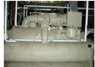
McQuay Centrifugal Chiller Unit
