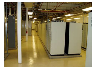
Power and UPS Room
