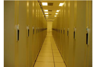
Data Center Floor – Server Cabinets
