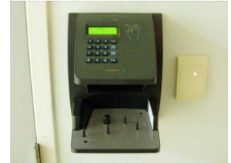
Biometric and Proximity Access Controls
